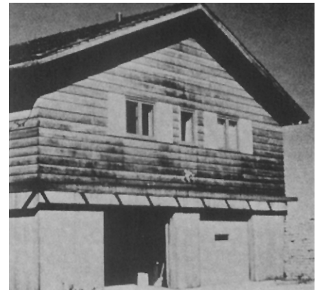
Figure 6. Mildew discoloration on house siding.
