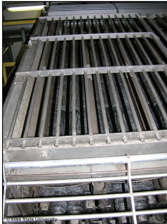
Figure 15. Rolls of a husking bed underneath safety grate
