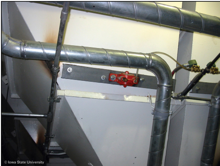
Figure 19. Pneumatically operated vibrator mounted on bottom exterior of storage bin
