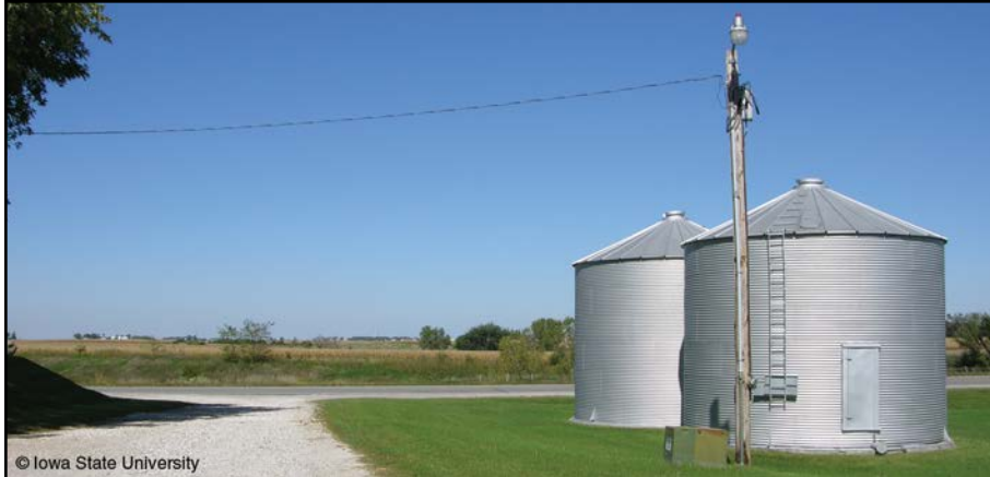
Figure 43. Overhead electrical lines at grain bin site
