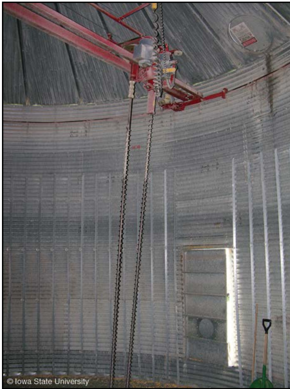
Figure 28. Vertical stirring augers suspended from overhead track inside a drying bin
