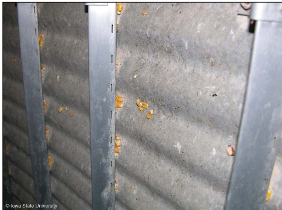
Figure 30. Vertical air tubes along interior bin wall
