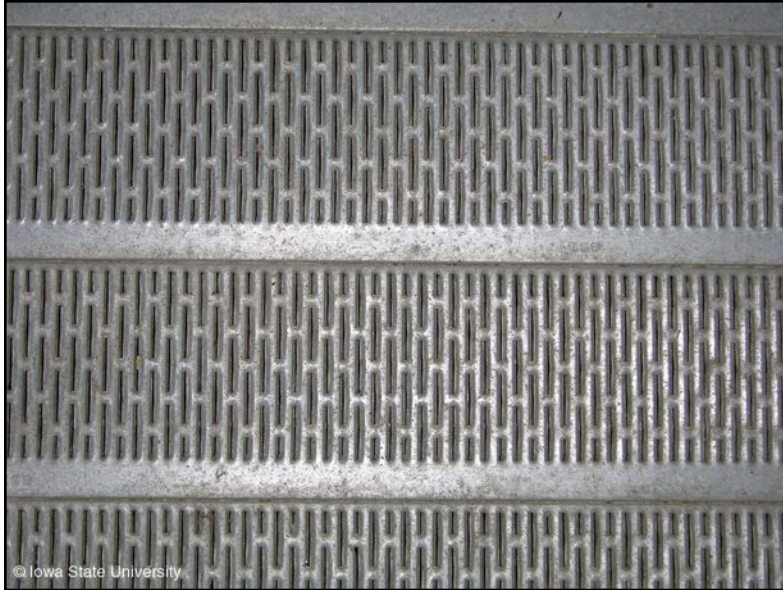
Figure 6. Perforated bin floor surrounding sump location
