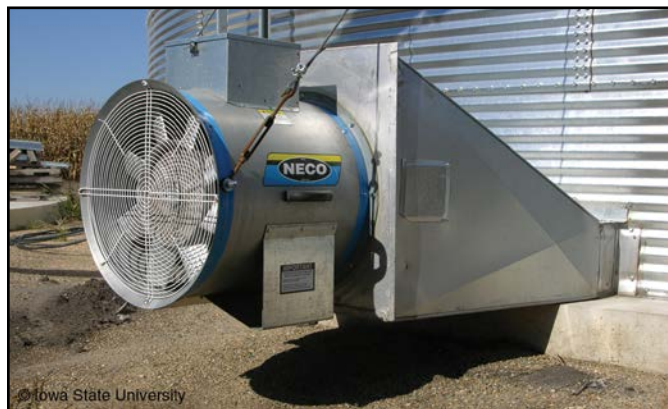
Figure 5. Fan on outside perimeter of bin
