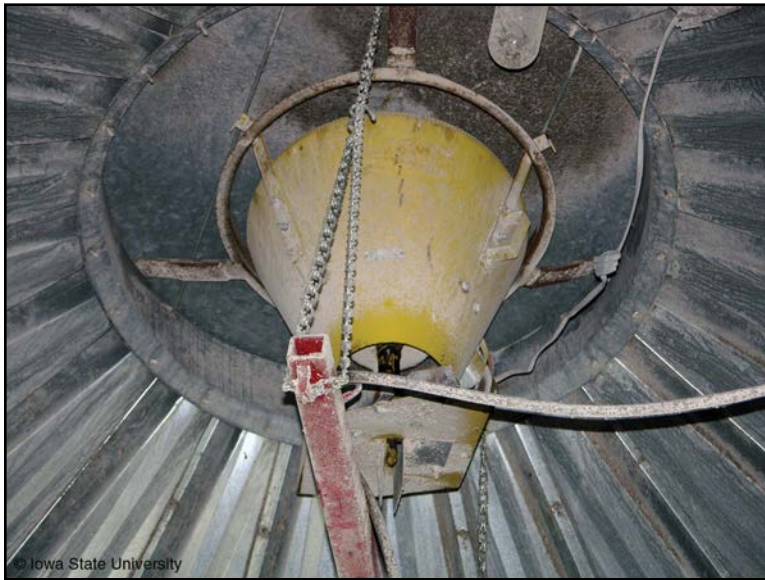
Figure 3. Grain spreader mounted in top of bin
