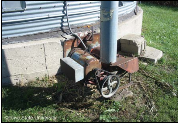
Figure 23. Conveyor junction point where horizontal auger under bin floor delivers grain to vertical unloading auger on side of bin (safety shield missing around belt drive)
