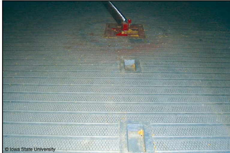
Figure 12. Auxiliary unloading sumps in bin floor over bottom unloading conveyor
