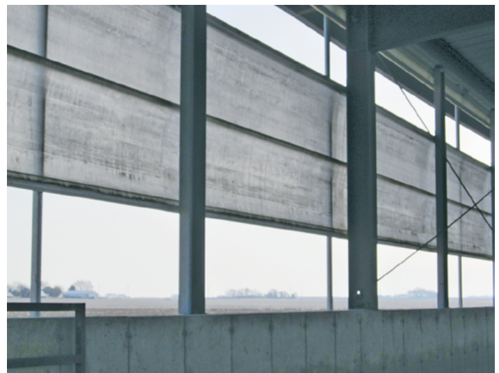
Partially closed curtain
