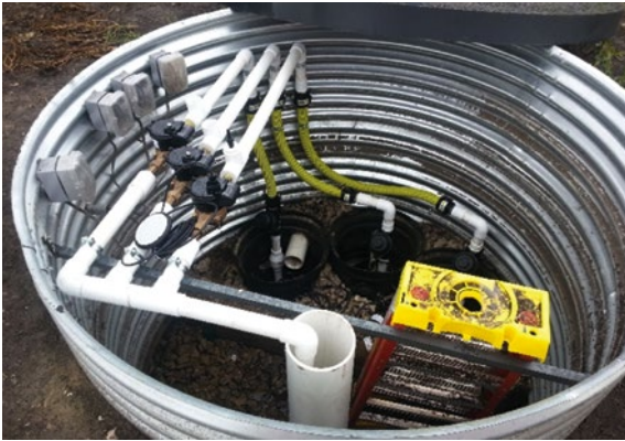
Figure 3. Pumped flow monitoring setup inside drainage monitoring sump at NWRP.
