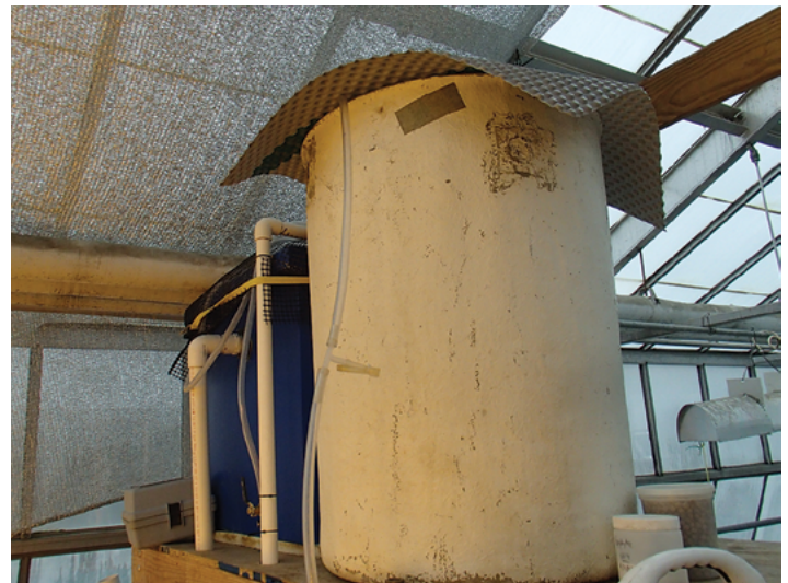
Figure 12. Head tank with covering to prevent algae.
