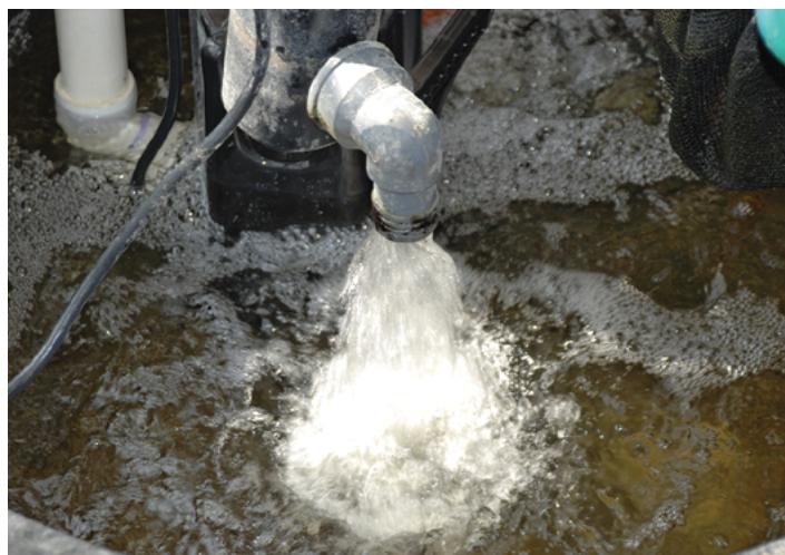
Figure 8. Submersible impeller pump with waterfall aeration.
