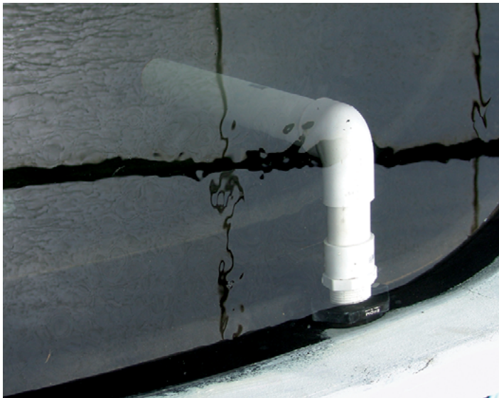
Figure 3. Solids lifting outflow.
