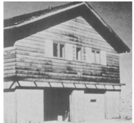
Figure 6. Mildew discoloration on house siding.
