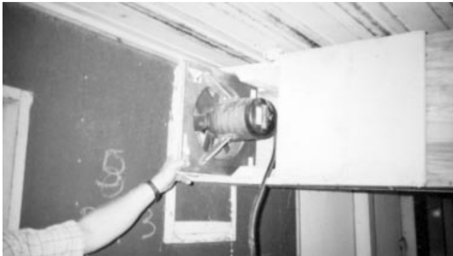
Photo B. The hinged access door (located to the right of the fan) allows you to manually turn around this fan, which does not have a reversible motor.
